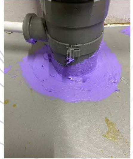
5.1.4 Soil stack through floor
