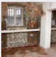
On damp masonry
