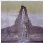
For water bearing cracks
