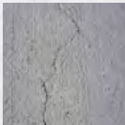
Penetrates into very fine cracks
