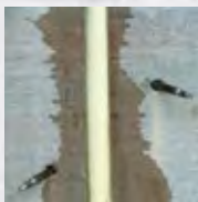
Forms foam in wet cracks
