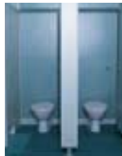
Cubicle with full height framed duct panel system
