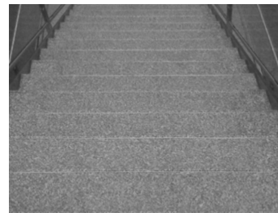
Poor Visual Contrast No Stair Nosings – Don't Take the Risk
