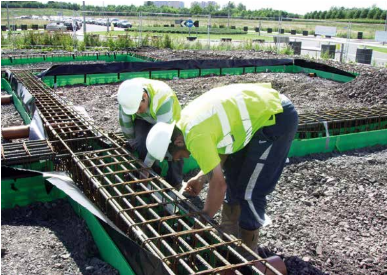
Fitting Proofex Total gas membrane starter strip, ready for connection to the under slab membrane
